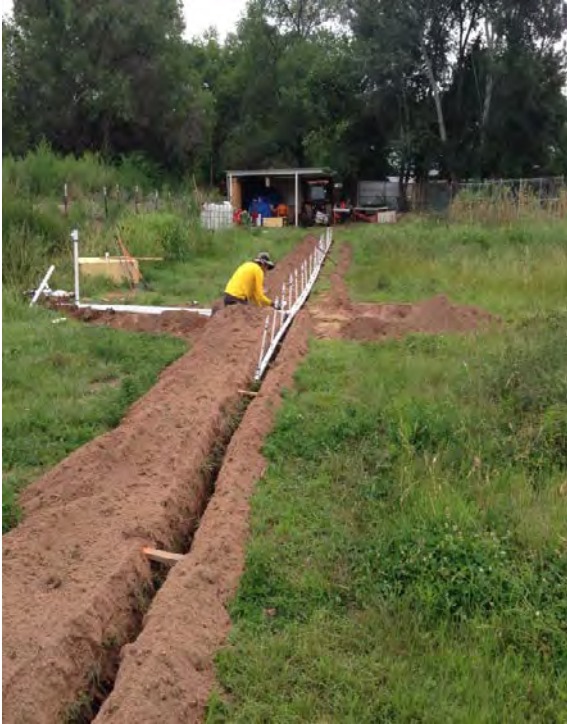
Permanently buried manifold and distribution lines
