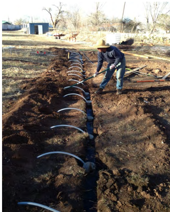
Irrigation lines spaced every 30"
