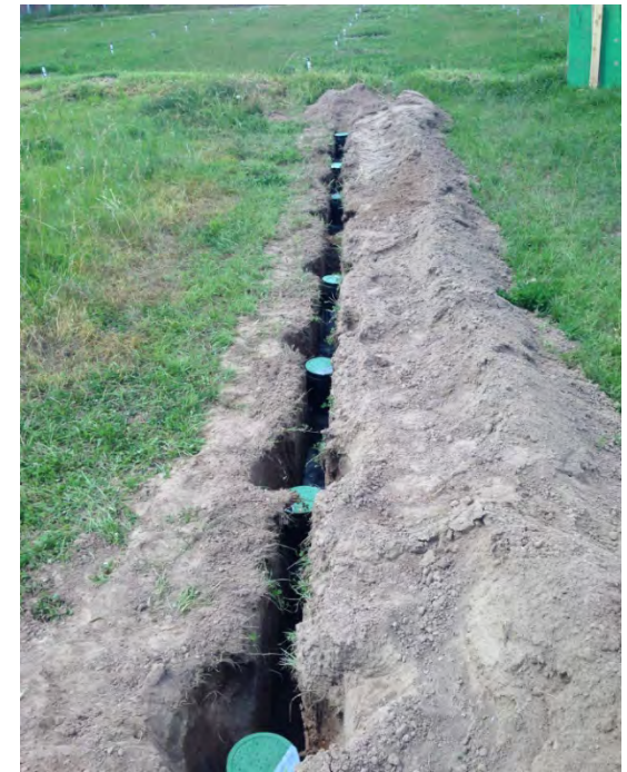
Every row has buried control box
