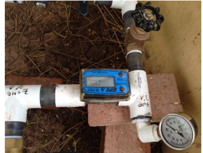
Flow rate meter and valves
