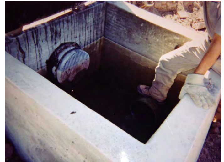
Finished water control structure
